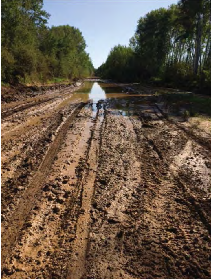
Figure 4 - Degradation of the road
